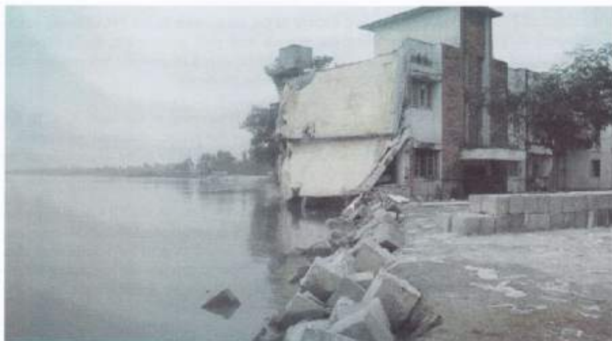
Picture-1. Chowhali Upazilla Officer's Quarter is collapsing and going under water due to river erosion.
