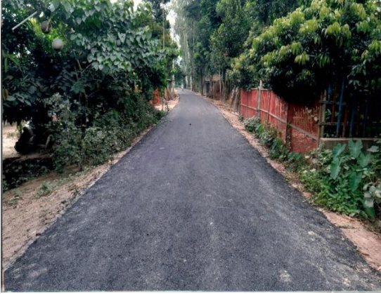
Periodic Maintenance of Nimgachi UP- Jorshimul Hat Via Majbari Road from Ch. 2194m- 5208m [ Road Id- 110273008 ], Upazila: Dhunat. Dist: Bogura.
