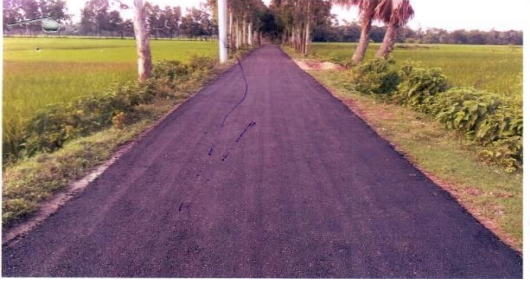
Periodic Maintenance of Adamdighi- Tilokpur Via Shalgram Road from Ch. 1100m- 5220m [ Road Id- 110062008], Upazila:Adamdighi, Dist: Bogura.
