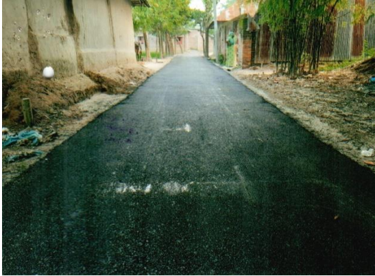
Periodic Maintenance of Gohail U.P- Atail hat Road from Ch. 2750m- 3800m [ Road Id- 110963001 ], Upazila: Shajahanpur, Dist: Bogura.
