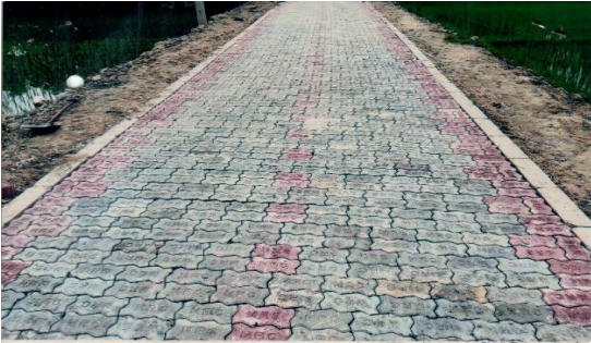
Rehabilitation of Shimulkandi School- Ram Narayanpur Road (via kanudasanganti) Road from Ch. 00m-530m under Dhunat Upazila, District: Bogura [Road ID # 110274033].
