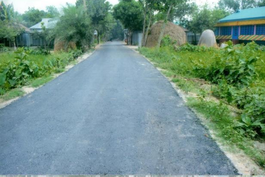
Rehabilitation of Mothurapur-Amir Bari Road-Hatlal village road via Naruli Gorostan Road from Ch. 00m-671m under Nandigram Upazila, District: Bogura
