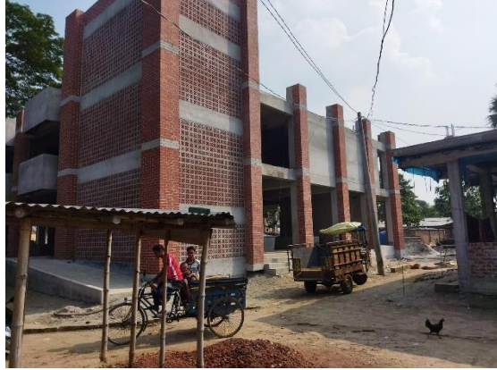
Construction of Two (2) Storied Rural Market Building (With 04 Storied Foundation) in Hatkaroy Hat, Under Nandigram Upazila, Dist.-Bogura.
