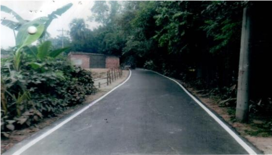
Periodic Maintenance of Sonahata GC- Toronihat GC (Dhunat Part) Road from Ch. 00m- 1980m [ Road Id- 110272007 ], Upazila: Dhunat. Dist: Bogura.
