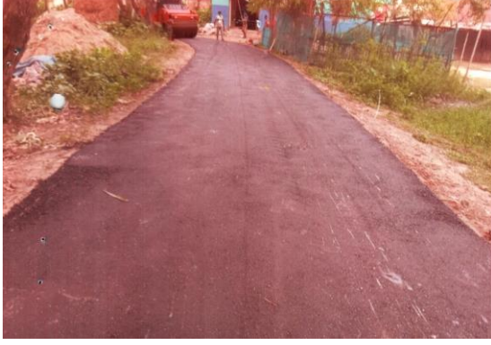
Periodic Maintenance of Bogra Natore Highway- kusta Road from Ch. 00m- 910m [Road ID-110675023] Upazila: Nandigram, District: Bogura.
