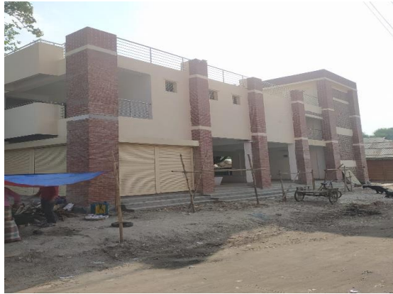
Construction of Two (2) Storied Rural Market Building (With 04 Storied Foundation) in Hatkaroy Hat, Under Nandigram Upazila, Dist.-Bogura.
